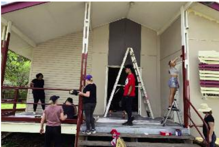
St Peter Claver College students and staff repairing the front of the St Peter Claver Chapel in Cherbourg.
